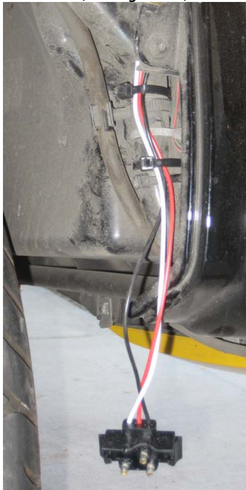
Figure 13. Wiring harness secured with cable ties.
