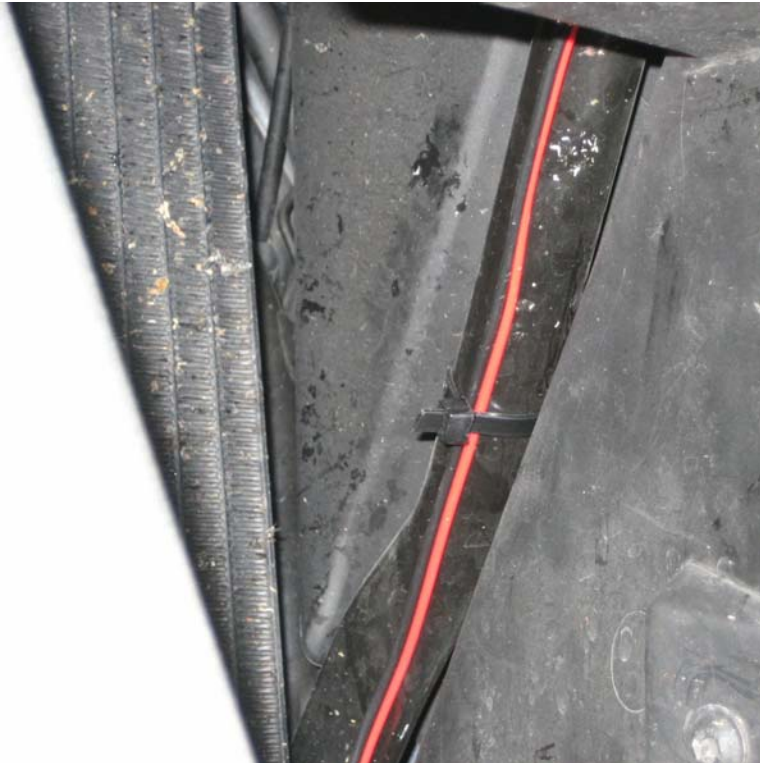
Figure 13: Zip cord fastened to frame with black cable tie
