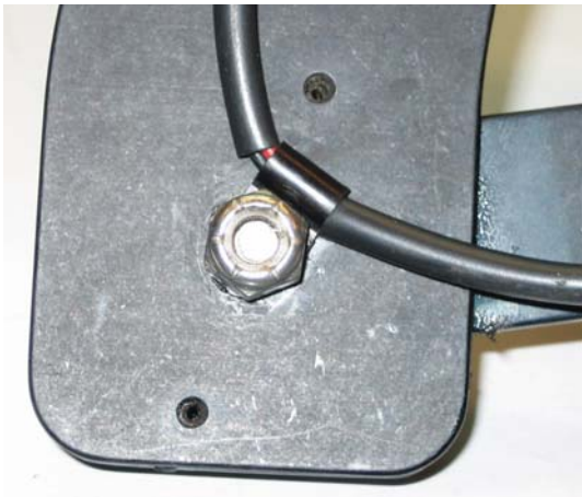
Figure 5: Close-up showing angle of cable clamp holding the wires
