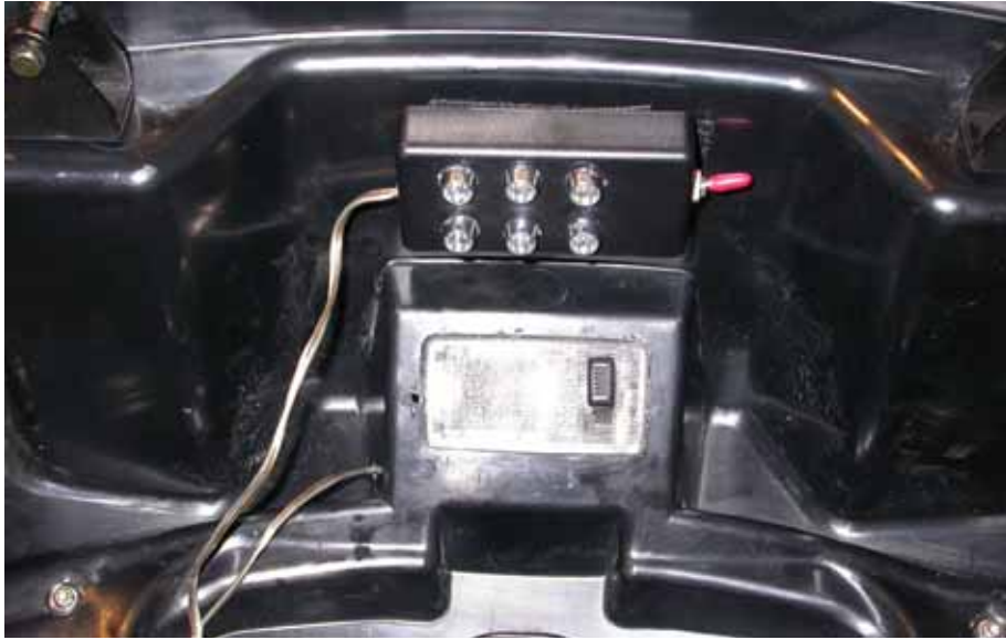
Figure 5. LED trunk light mounted to the top of the trunk
